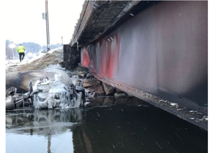
Fig. Bridge-129 after fire.
