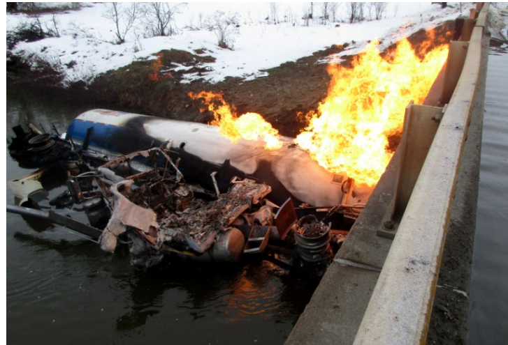
Fig. Bridge-129 during fire.
