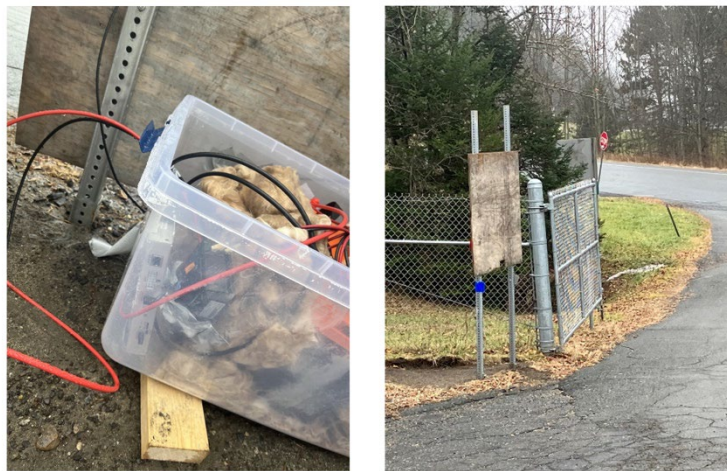
Fig. 19: storage box and two poles for mounting antennas
