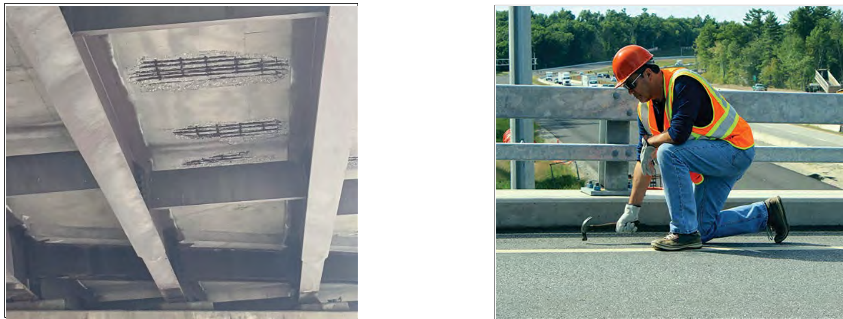
Figure 1. Delaminated Underside of Bridge Deck (left) Technician Uses Hammer to Inspect Bridge (right)
