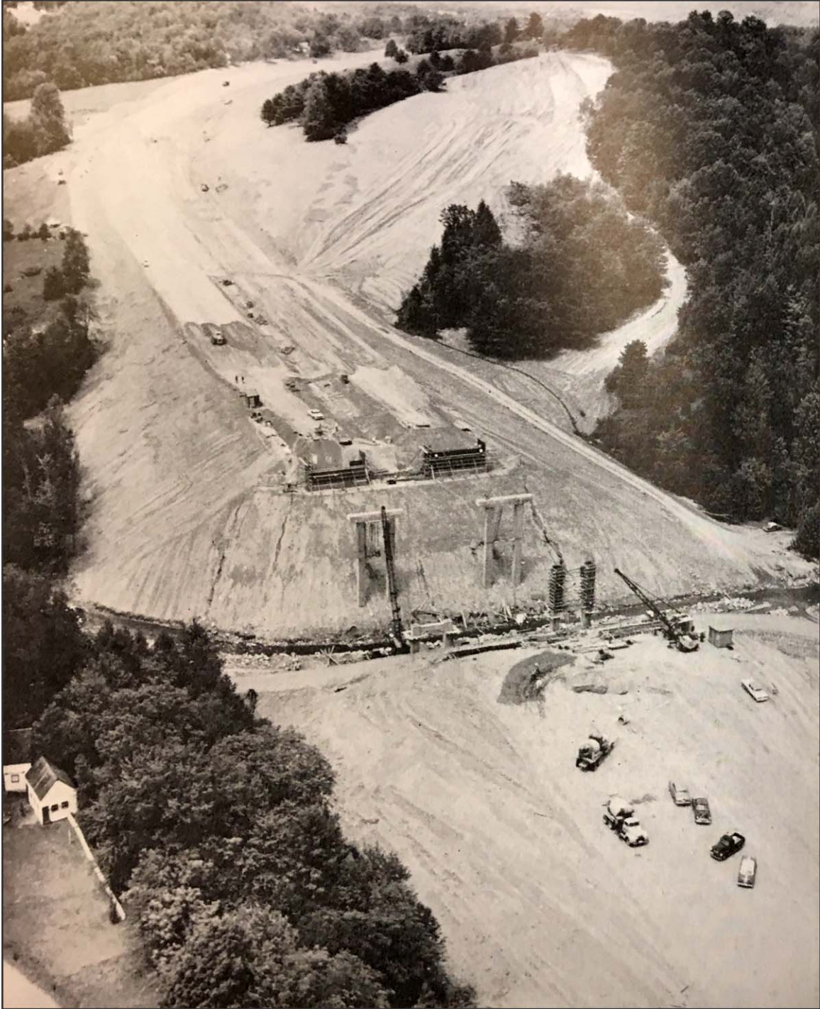
FIGURE 8: Construction of Twin Bridges over Broad Brook on the Brattleboro Bypass (Vermont State Highway Board 1956-1958)
