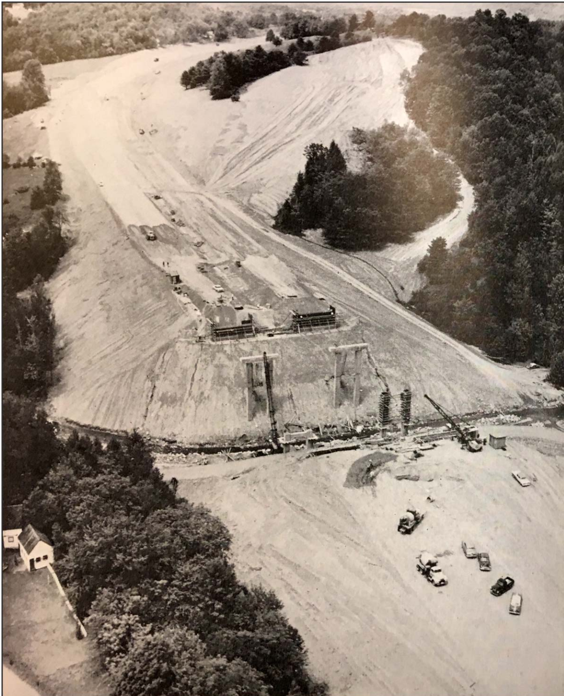
FIGURE 3: Construction of Twin Bridges over Broad Brook on the Brattleboro Bypass (Vermont State Highway Board 1956-1958)
