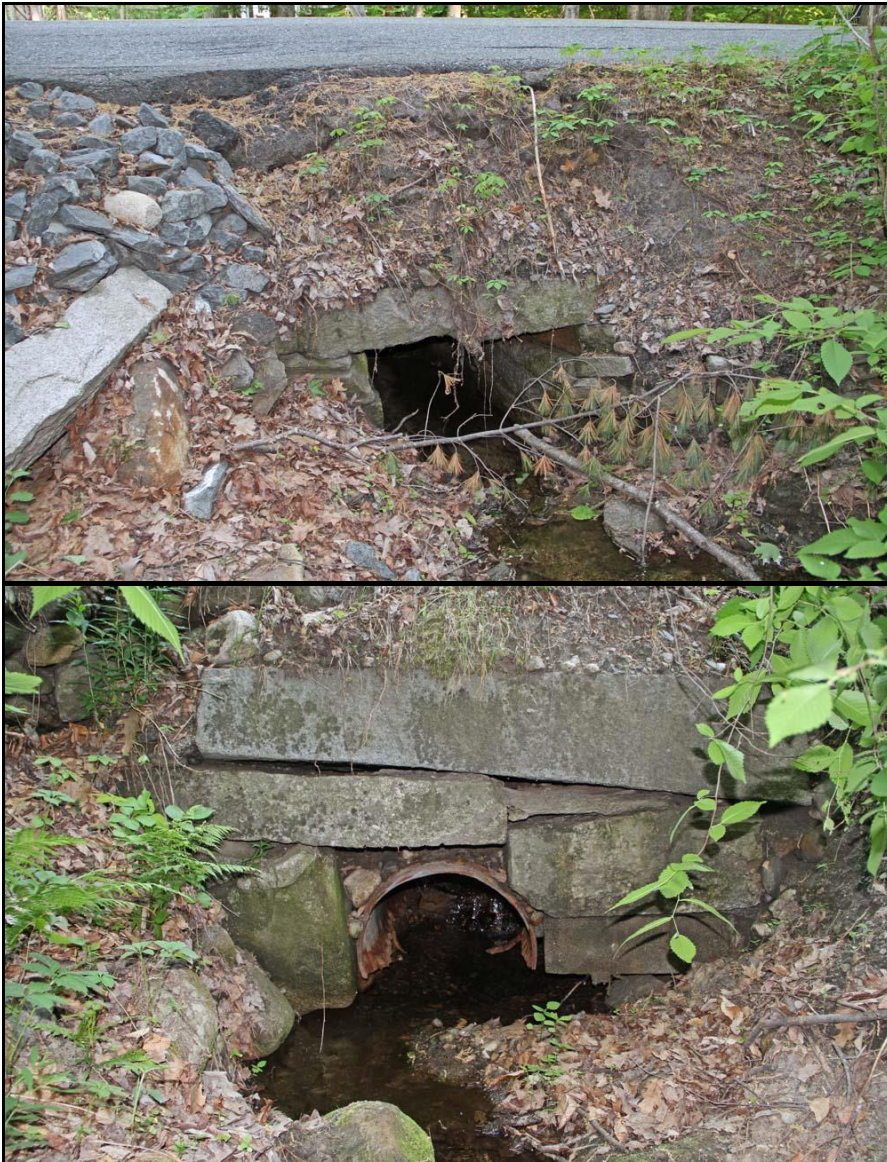
FIGURE 15: Upper Dummerston Road, Dummerston (WI-DUM-003). Lengthened with pipe. Upstream end as originally built, top photo; downstream end showing steel pipe and stone probably salvaged from old facewall and reused.
