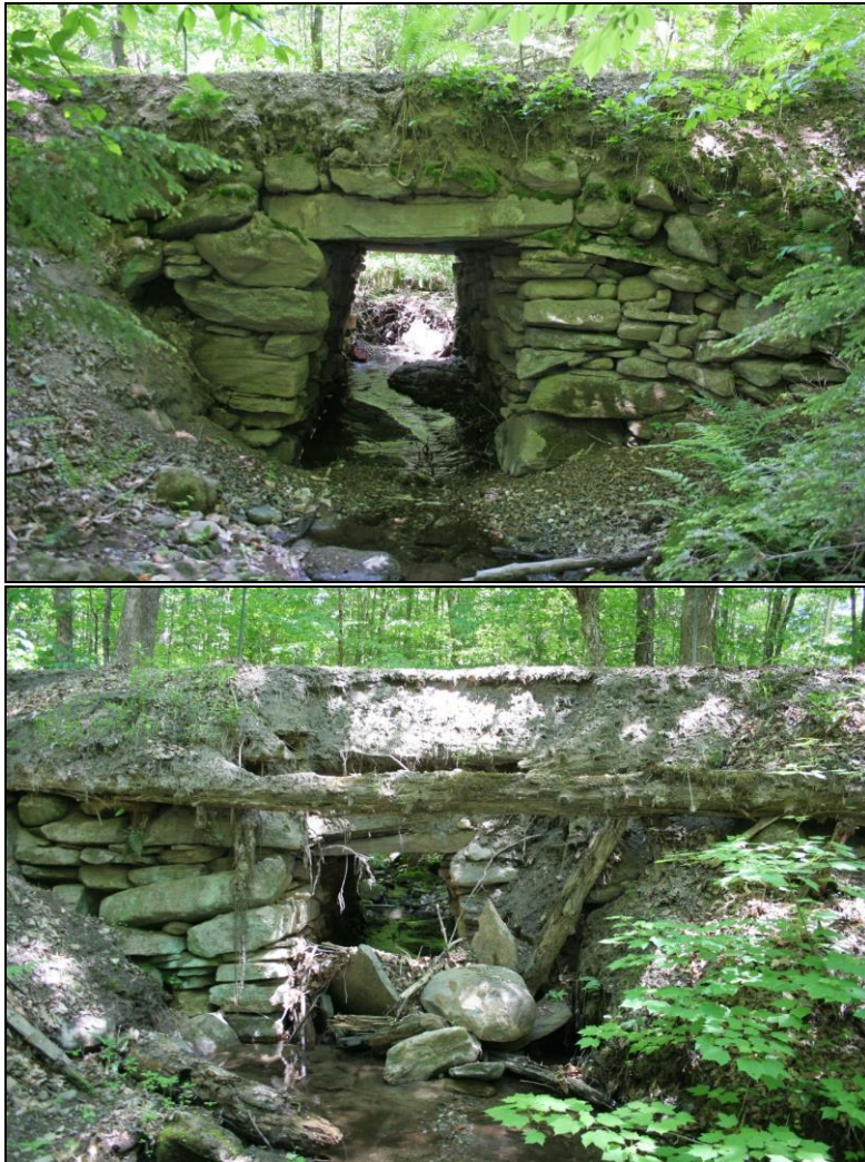
FIGURE 14: Deer Ridge Road, Townsend, (WI-TOW-001). Partial collapse.
