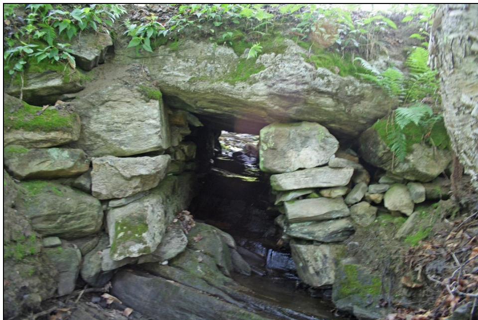
FIGURE 10: Goldwaite Road, Chester (WN-CHE-008). This field and rubble stone box culvert was built on a stream bed of exposed ledge, an ideal foundation were it not sloping. The "downhill" channel wall was not given sufficient buttressing and has slipped to the point of imminent collapse, in part due to the oblique loading of the massive cover stone.
