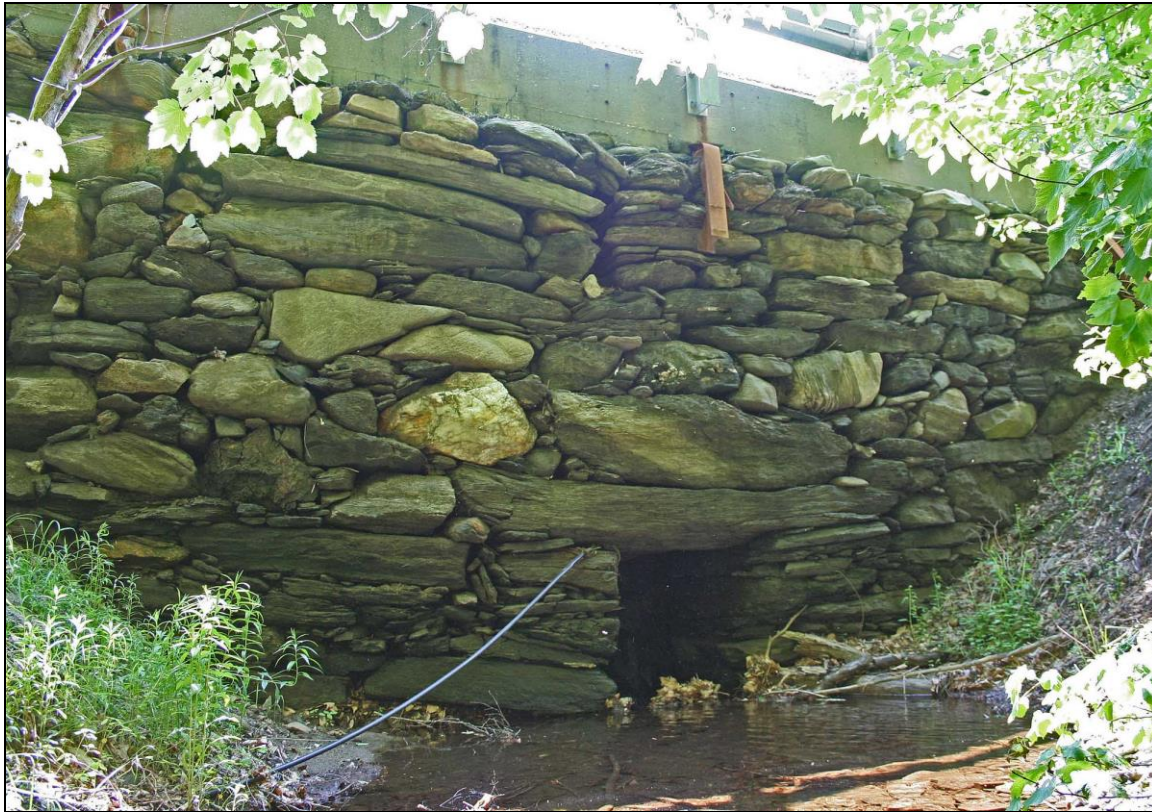
FIGURE 7: This extraordinary box culvert in on Windham Hill Road in Windham (WI-WIN-001), has a large area of waterway opening, with a 54" opening width (span) and 102" opening height. It is built entirely with fieldstone, some of astounding size that would have required several oxen to move and probably an A-frame derrick to place. The upstream facewall reaches a total height of over 25 feet. When the highway was widened, the culvert was lengthened with the addition of a concrete box structure and concrete block facewall on the downstream side, shown in Figure 17 below.
