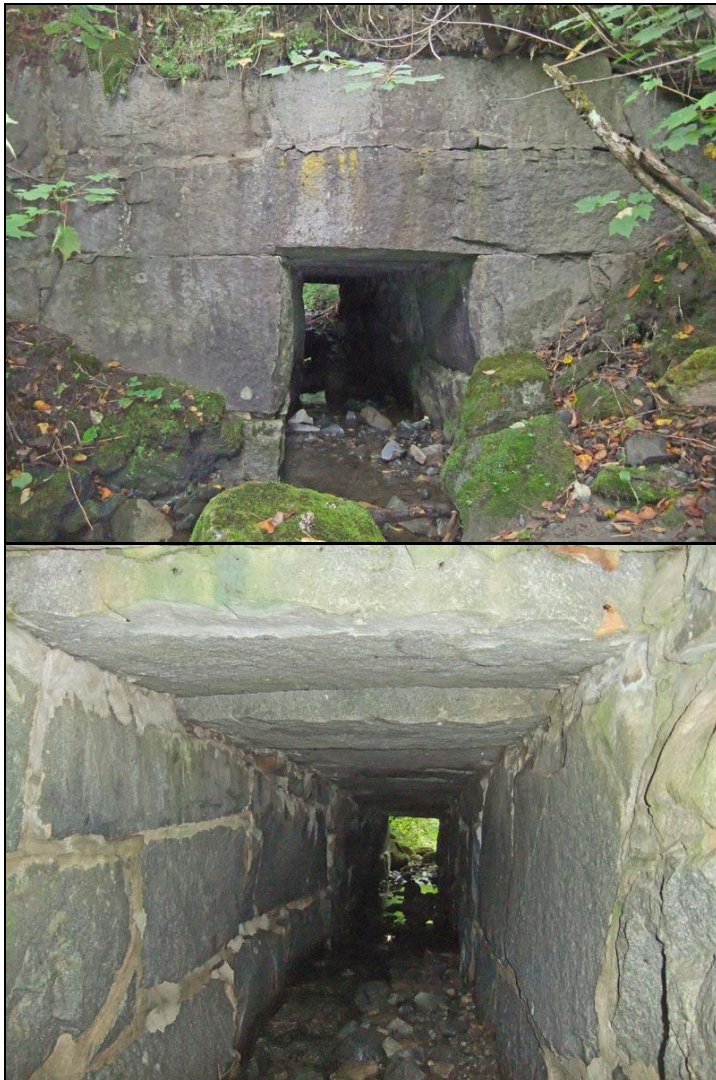
FIGURE 18: Royalston Corner Road, Concord (ES-CON-001). Box culvert of cut stone laid in mortar.
