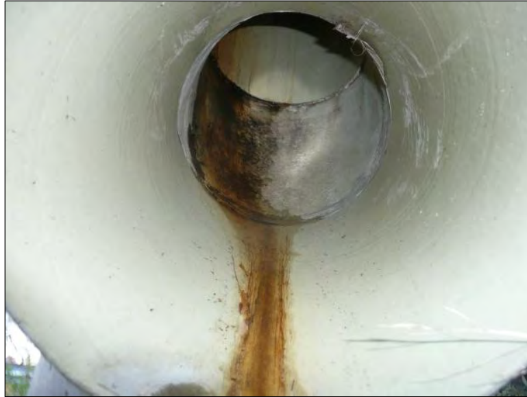
Figure 4 - Iron Oxide Discoloration 2010
