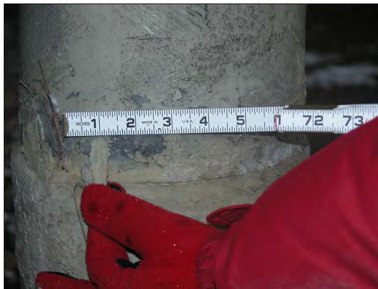
Figure 1 – Flaking of Adhesive
