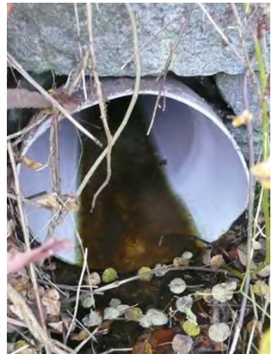
Figure 7: 18-inch pipe outlet, 2010
