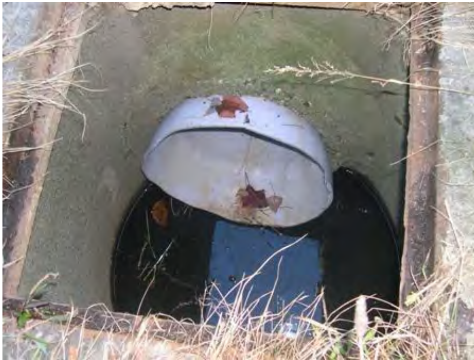
Figure 9: Photograph of the inlet of the 18-inch liner in 2004.
