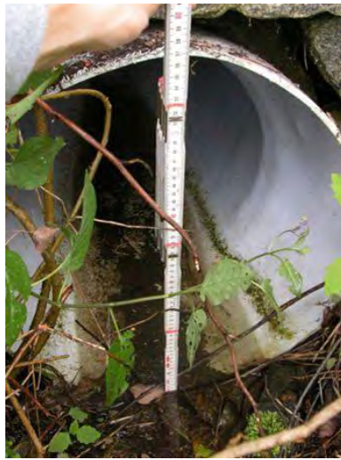
Figure 6: 18-inch pipe outlet, 2007
