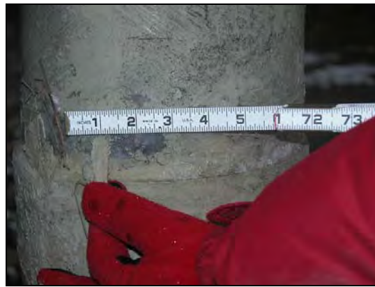
Figure 3 – Flaking of Adhesive
