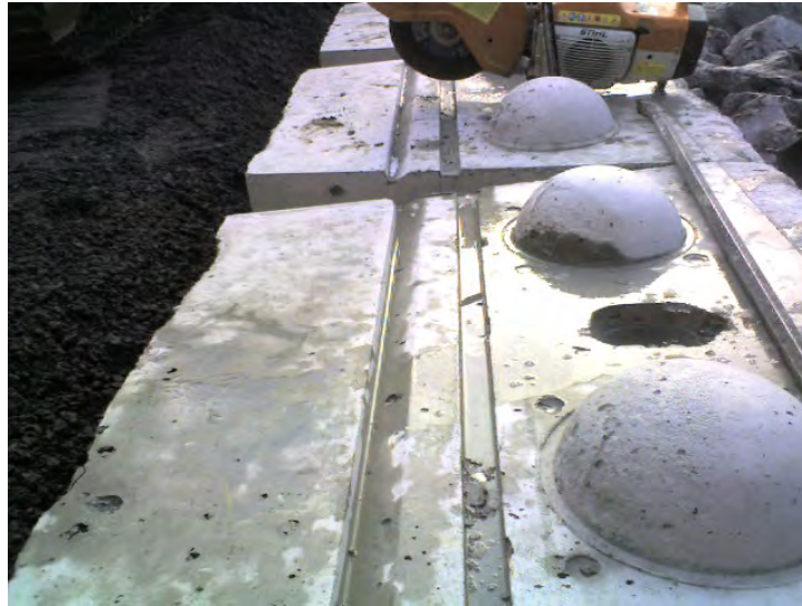
Figure 8: Reinforcing steel channels out of alignment
