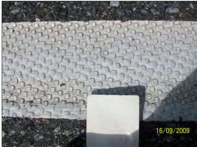
Figure 5. Appearance of the 3M Series 380WR ES tape 328 days post-installation.
