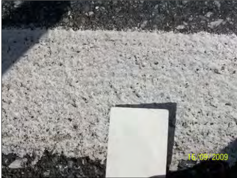
Figure 6. Appearance of the 3M LPM 1200 polyurea 325 days post-installation.
