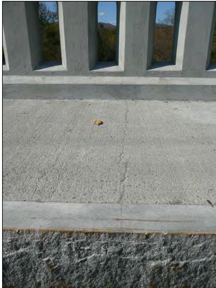
Figure 17. Cracking in Randolph rail, sidewalk, and curb.
