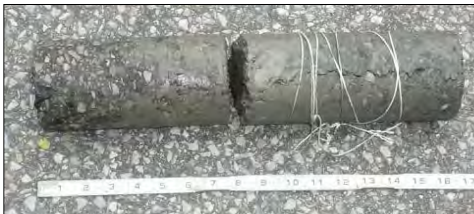
Figure 6 Core Extracted Over Crack
