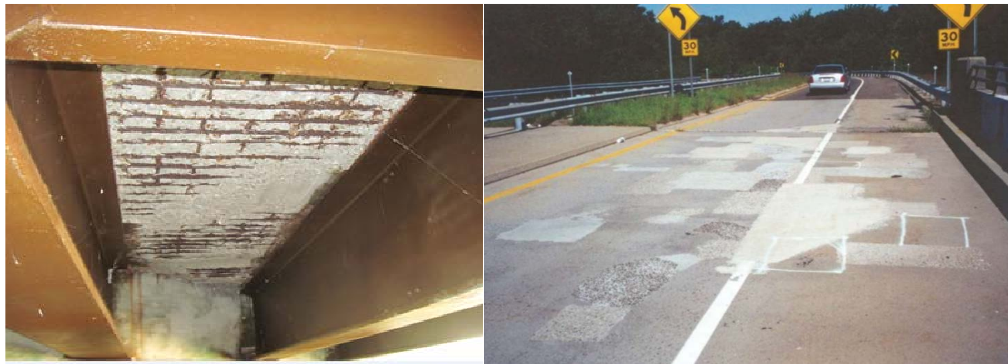
Figure 1. Bridge Deck Delamination caused by chlorides
