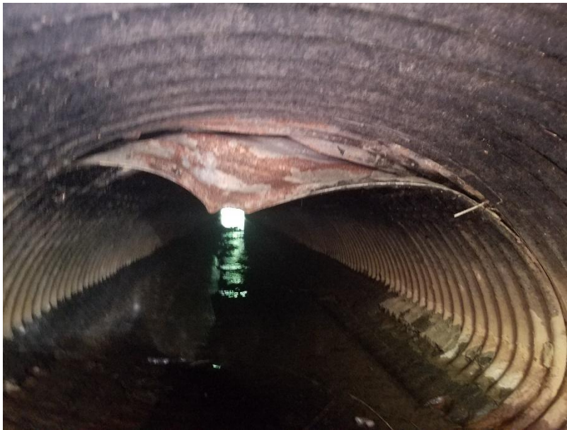
Figure 1 Photo Showing Vermont Culvert in Need of Repair (Initially Captured by Vermont's HIVE in May 2018)
