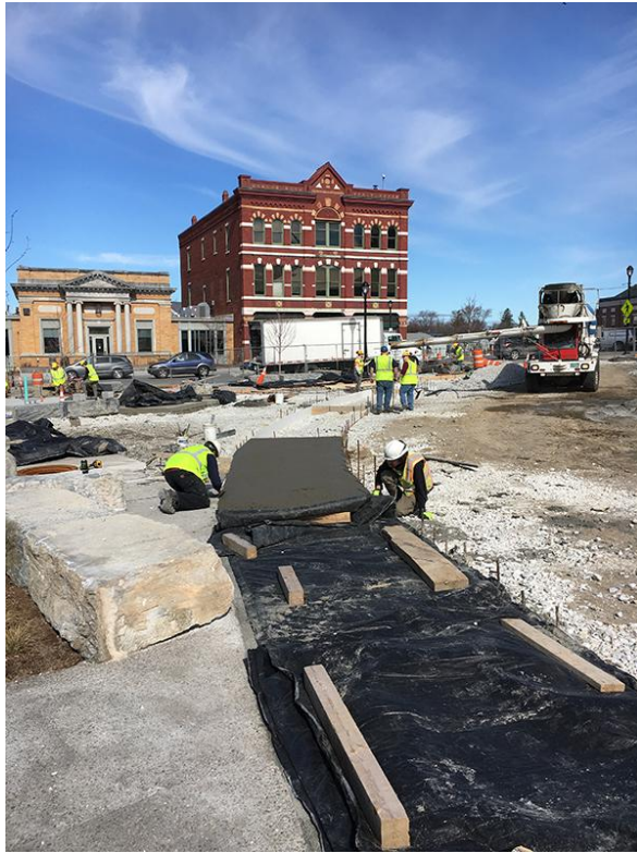
Contractor Waters Excavation pours sidewalk panels in Triangle Park. They will finish pouring concrete as early as next week.
