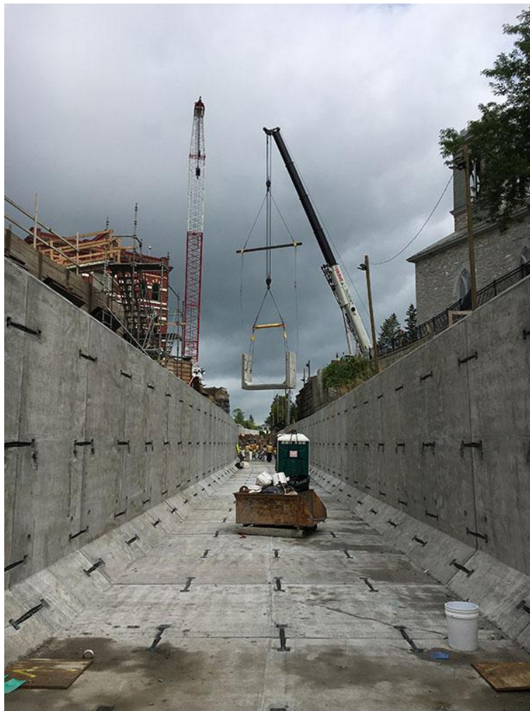
A crane lifts one piece of concrete u-wall to set it into place.
