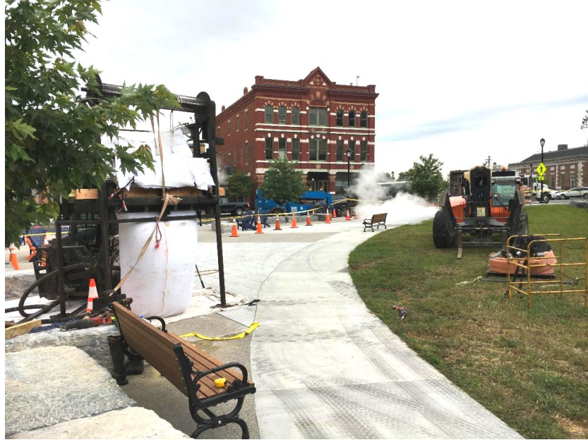
Crews install a fiberglass liner in one of Triangle Park's new storm pipes.
