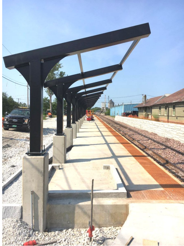
The rail platform on the north end of the project is nearing completion.
