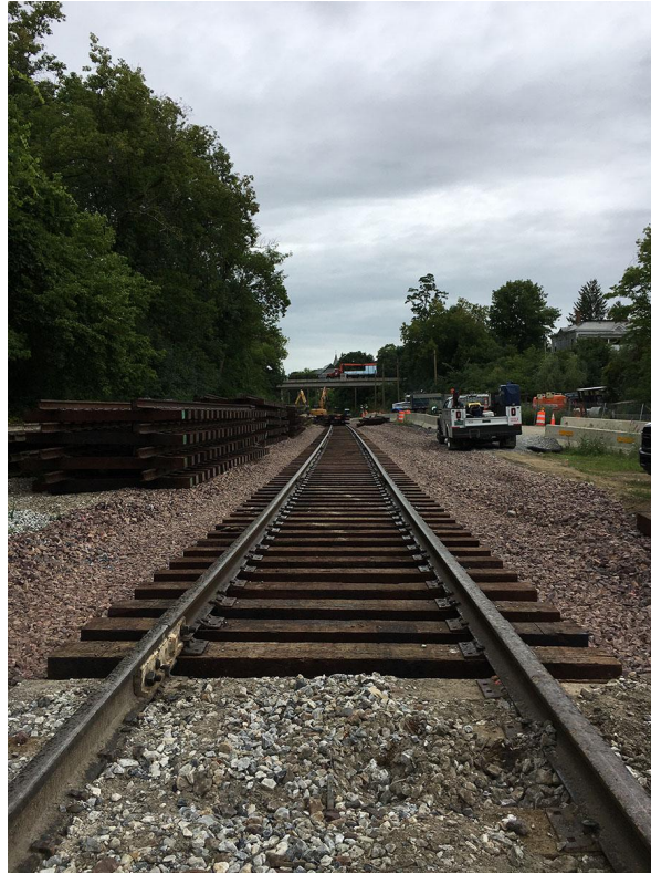
Taken from the trestle bridge across Otter Creek at Water Street, the image above shows the panelized rail track sections in place on top of the ballast stone.
