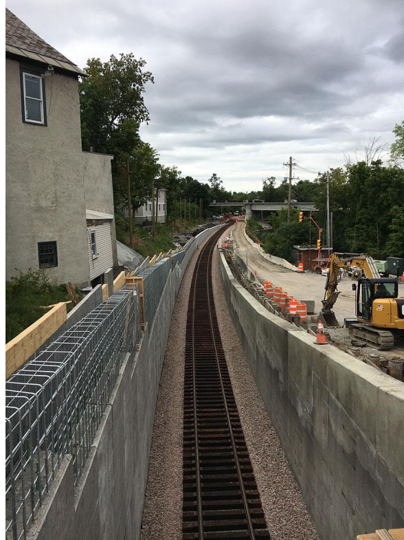
Patriot Shotcrete formed the southwest cap wall, which you can see on the right in the photo. The southeast cap wall, formed to the left in the photo, will be shotcrete next week, along with northern sections of the cap wall.
