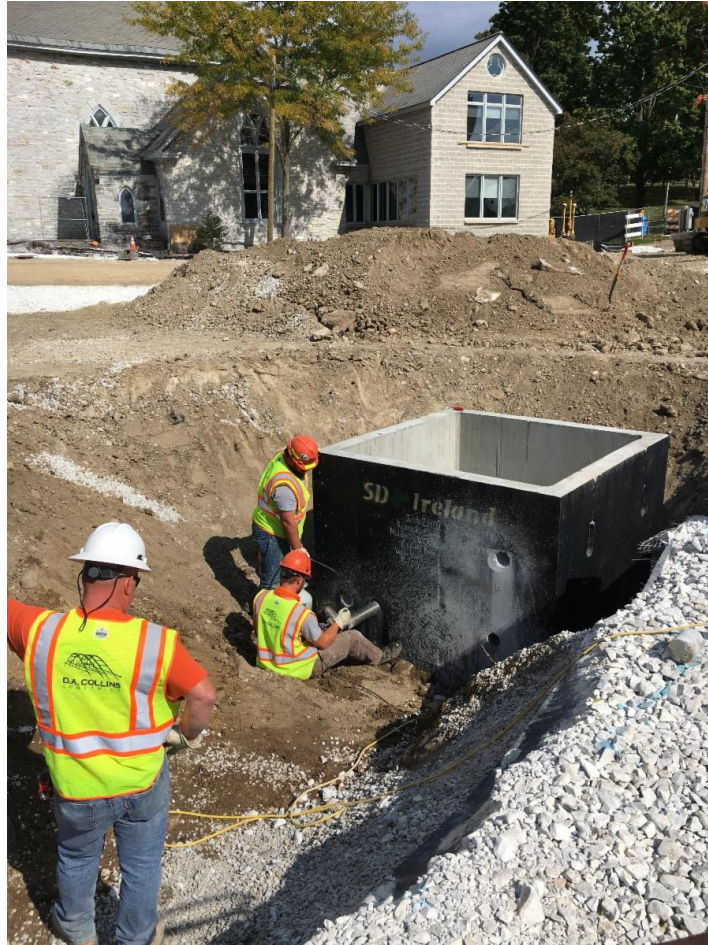
Above, Kubricky prepares a drainage pipe in a concrete water vault that will sit under Triangle Park. It will control operation of the park fountain.
