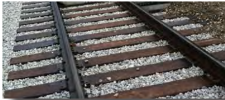
The condition of ties and ballast (crushed stone bed) are factors that determine weight capacity. Pictured here is a Vermont rail bed restored after a washout.
