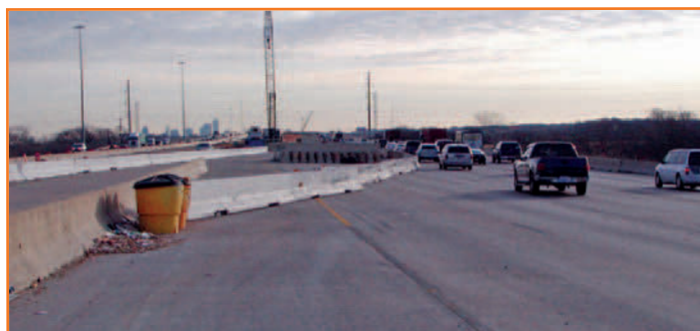
Barrier ends in work zones must be protected by flaring them and/or providing crash cushions (Source: TTI).
