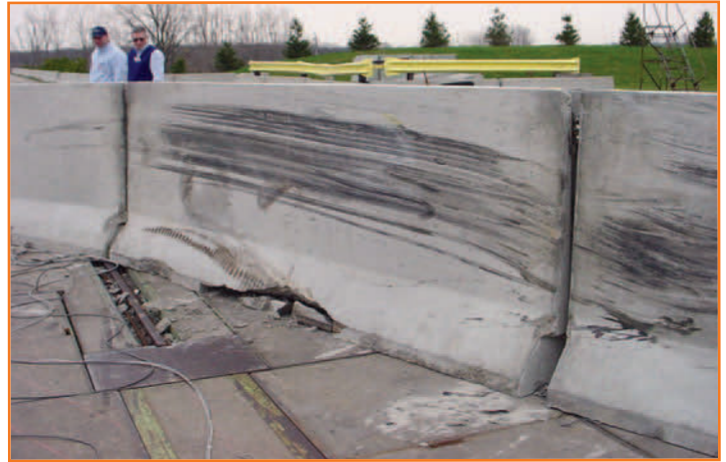
Workers should be aware that barriers can deflect when hit by an errant vehicle (Source: TTI).
