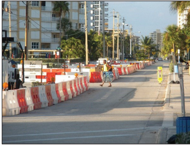
Figure 5. Example of longitudinal channelizers used to separate pedestrians from work spaces (source: TTI)
