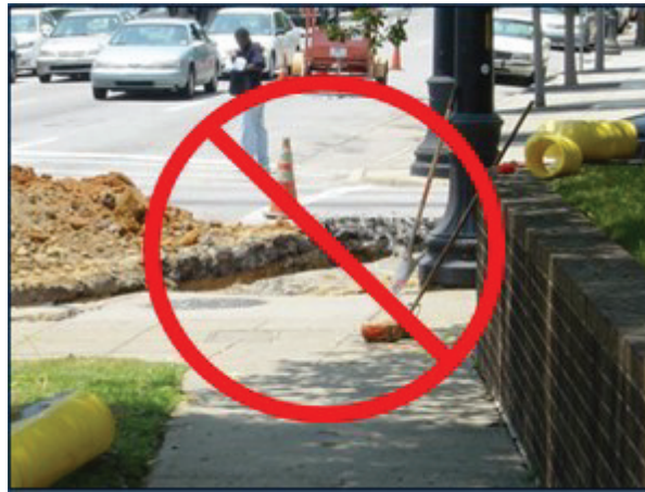
Figure 1. Open holes and trenches on or near pedestrian routes must be protected (Source: TTI)
