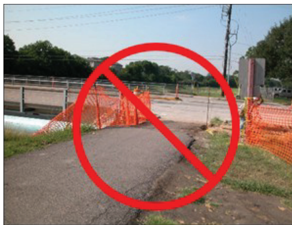
Figure 2. Mesh fencing is not sufficient to protect a pedestrian from falling into a trench or hole (Source: TTI)
