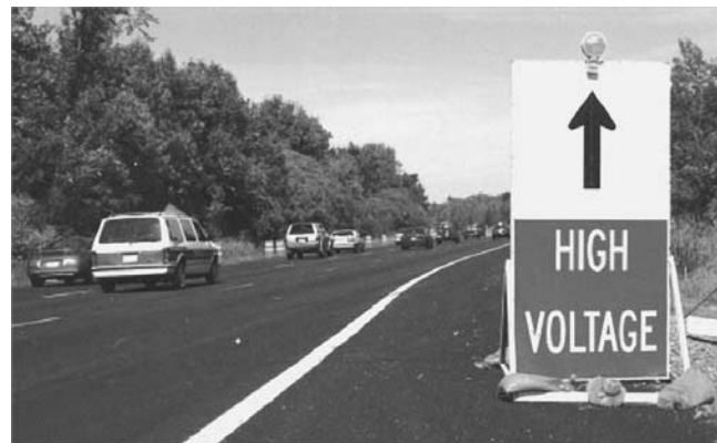
Figure 37. Portable sign with warning light.
