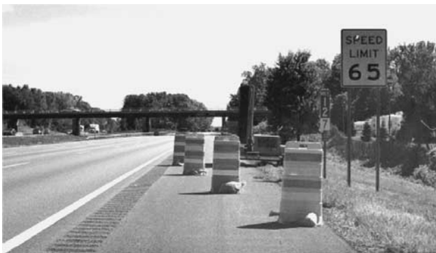
Figure 16. Properly shut down changeable message sign.
