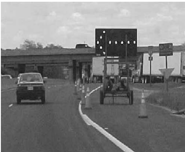
Figure 17. Preferred arrow panel location on the shoulder at the start of the taper.
