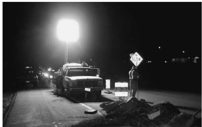
Figure 30. Glare aimed at oncoming traffic.
