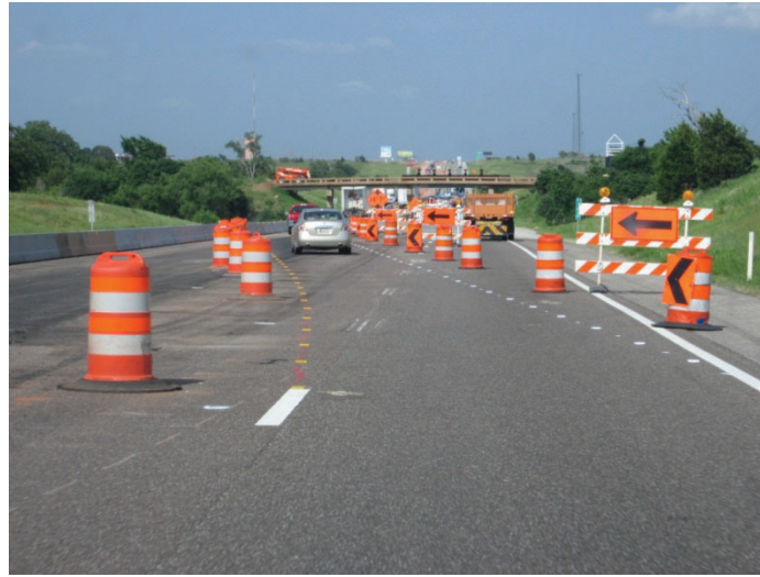
Figure 4. Use of Temporary Raised Pavement Markers on Lane Shift on I-44 in Oklahoma.
