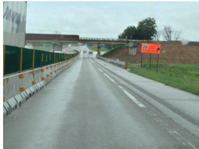
Figure 9. Use of Tabs on Barrier and Paint Wear on Edge Line on I-44 in Oklahoma
