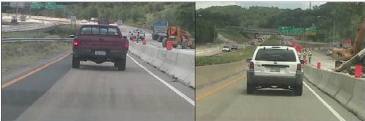
Figure 7. All-weather Pavement Marking (left) and Standard Pavement Marking (right) Work Zones on US-32/33/50 Eastbound in Ohio (Daytime).
