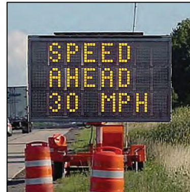
Figure 16 – PCMS in Work Zones Displaying Information about Conditions Downstream 9
