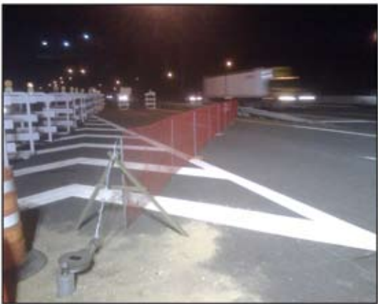
Figure 5. Vehicle Arresting System Protecting Closed Highway Section
