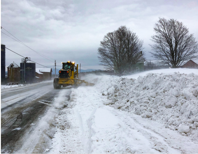
FRANKLIN. Even after a winter storm is over and snowplows have cleared a roadway, our maintenance crews stay busy. A crew pushed back snowdrifts caused by wind gusts along VT Route 120.
