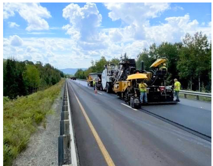
LYNDON-BARTON. A 40-mile interstate paving project began along I-91. Spanning three exits, work will also include guardrail replacement and drainage improvements.
